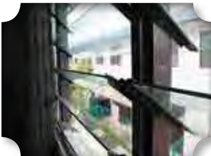
Australian adjustable glass louvered windows to facilitate air flow and ventilation
