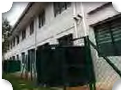
Rainwater harvesting tank for gardening and car porch washing without using potable water
